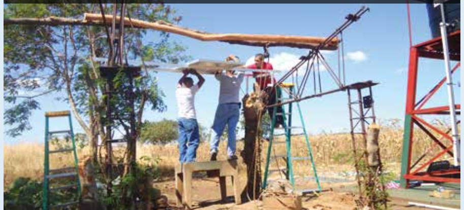
Installing solar panels to provide power to pump water from the well to the tank to supply water to the community and irrigate crops
